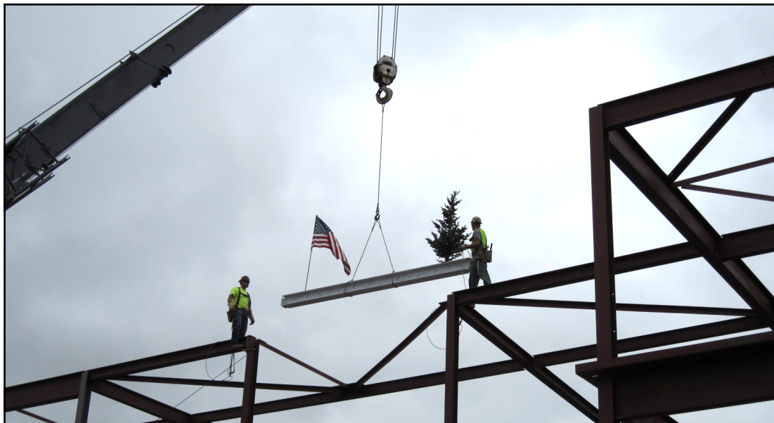
On August 23, 2010, the final beam was hoisted into place at the John and Marnie Demmer Wellness Pavilion and Dialysis Center. The facility will begin to serve patients in July, 2011.
